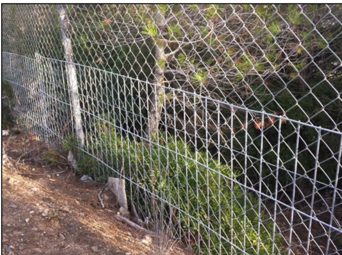
Reinforced welded mesh fence.
